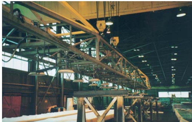
Bridge truss type unit used by a major aluminum producer to load finished aircraft wing skins into shipping container.
